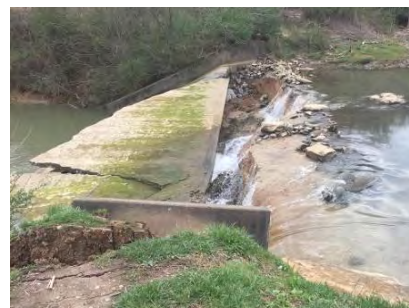
Auxiliary Spillway Failure
